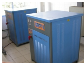
Figure 12. Hydrogen and oxygen generators on their installation site
